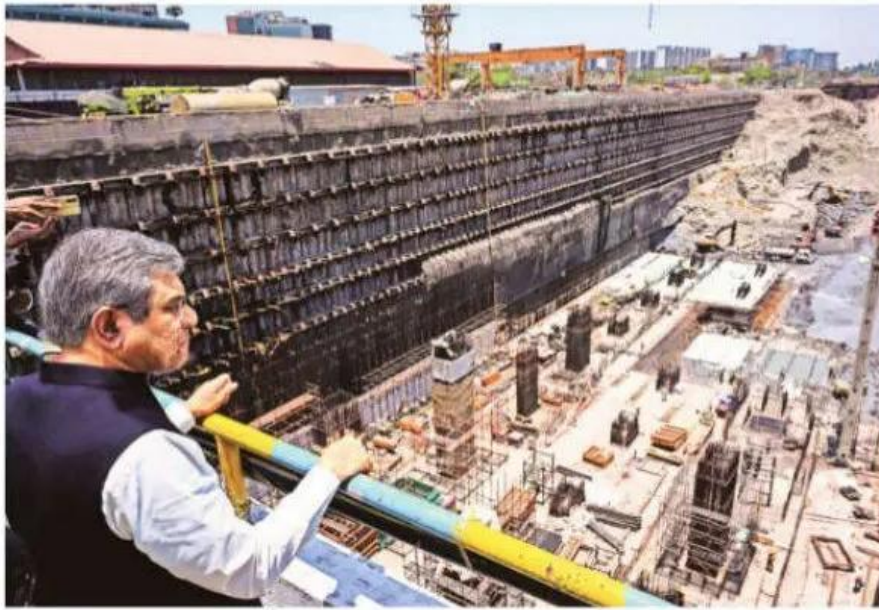
Railway Minister Ashwini Vaishnaw visits the underconstruction site of the Bullet train's station at BKC in Mumbai on Saturday. Sankhadeep Banerjee
